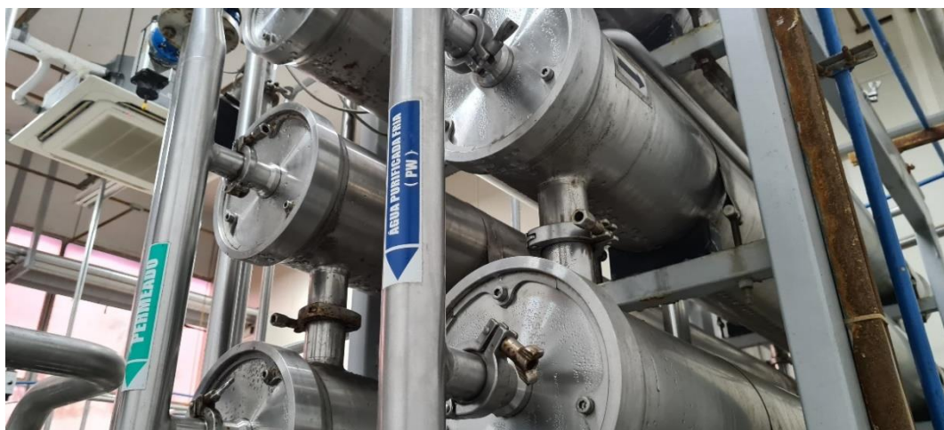
Water purification systems in our Production site of Suzano, Brazil
