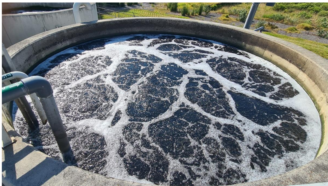
Wastewater Treatment Plant in our Vaccines Production site of Ocoyoacac, Mexico
