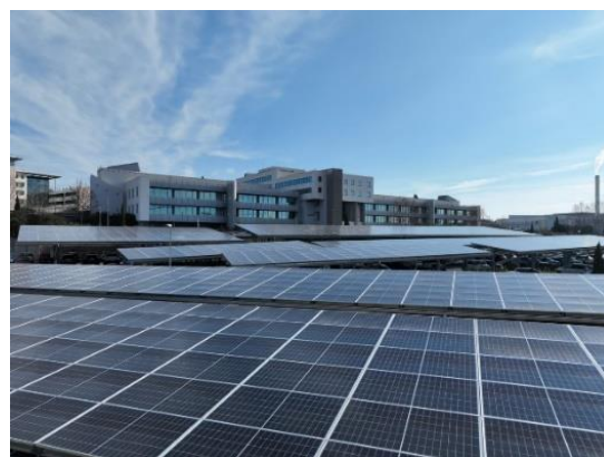
Solar panels in Montpellier site
