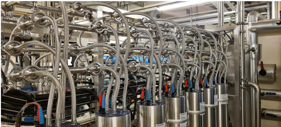
Water purification systems in our Production site of Val de Reuil, France
